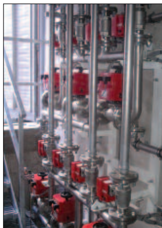
Prefabricated motorised valve manifold.
