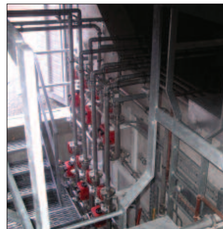
View down onto the valve manifold. Two storage tanks are to the right, but hidden.
