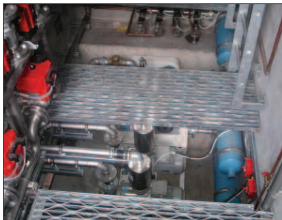
Beneath the grated floor are vacuum pumps, macerators and vacuum tank.
