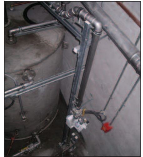
One of the storage tanks.
